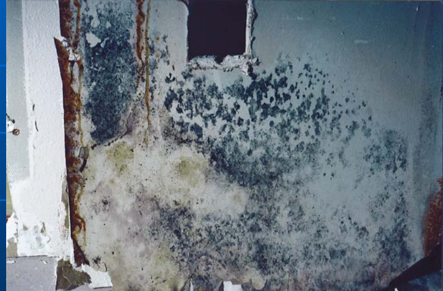
Interior cavity with hidden visible mold
