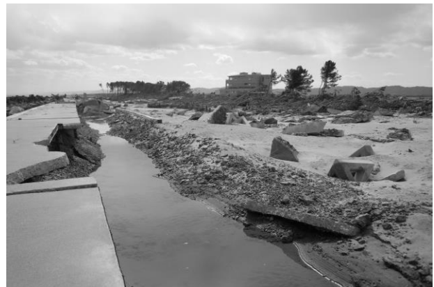
Fig. 5 Extensive failure of coastal dykes
