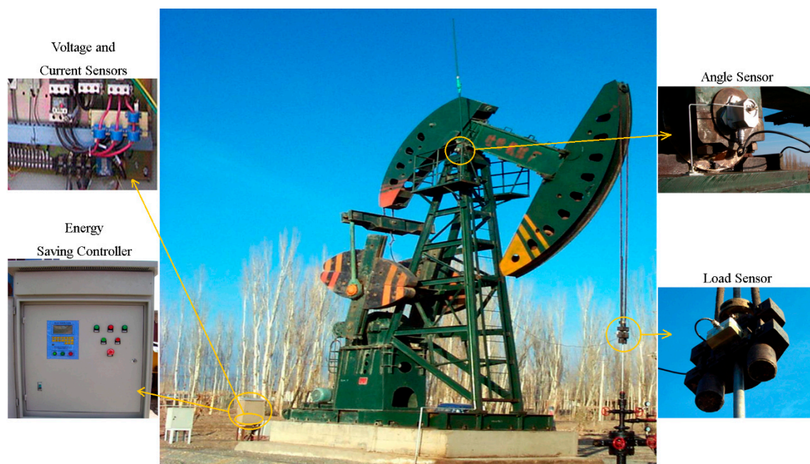
Figure 5. The energy saving device installed on a beam pumping unit, with the actual assembled positions for the four types of sensors and the controller.
