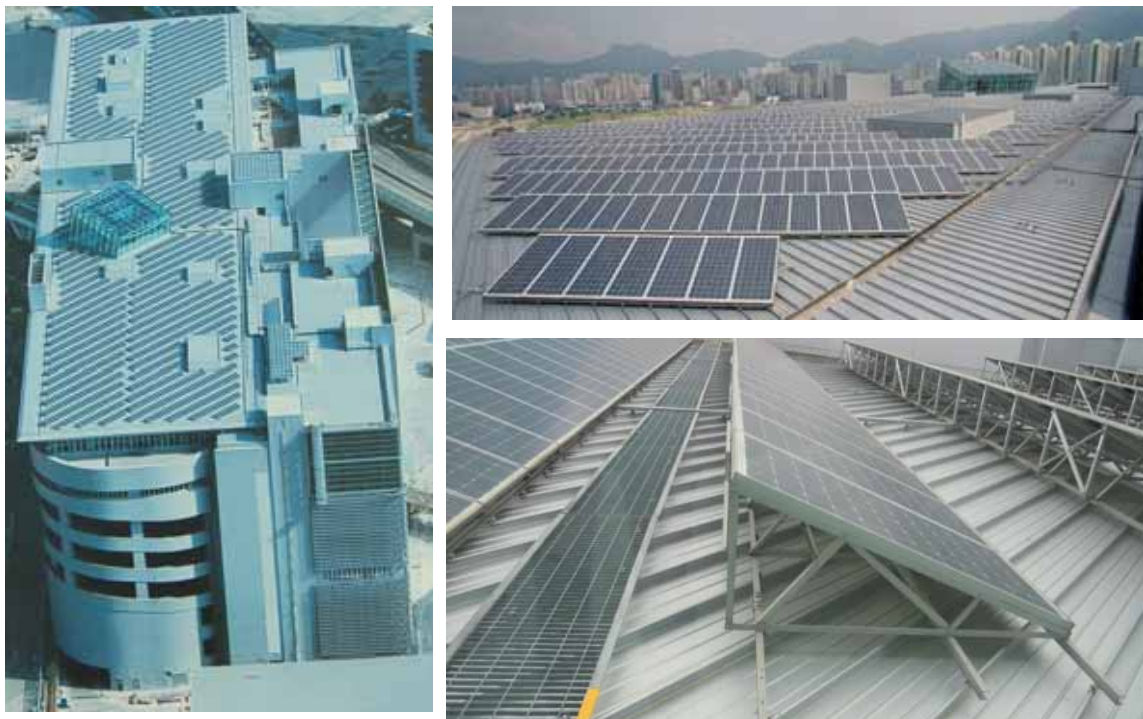
Figure 10. PV and roof systems at the EMSD Headquarters
