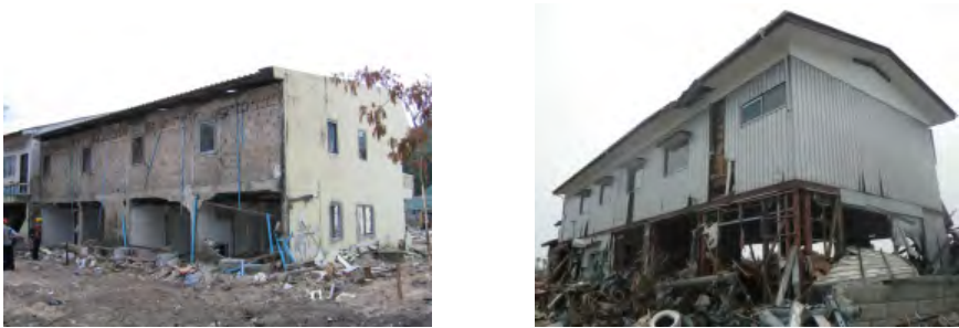
Fig. 25. Examples of building damage in the case of the 2004 Indian Ocean tsunami in Thailand and the 2011 Tohoku tsunami in Japan
