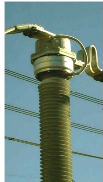
Figure 5 - FOCT metering installation at 132 kV mounted on top of the digital optical voltage transducer
