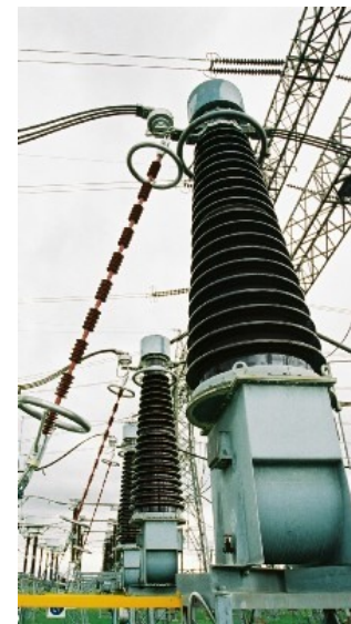
Figure 4 - FOCT Protection Installation on the 330 kV feeders with fibre-optic downlinks
