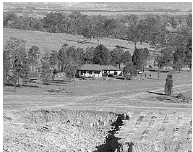
Fig. 2. Rix's creek house shown in background with section of overburden (foreground) ready for detonation
