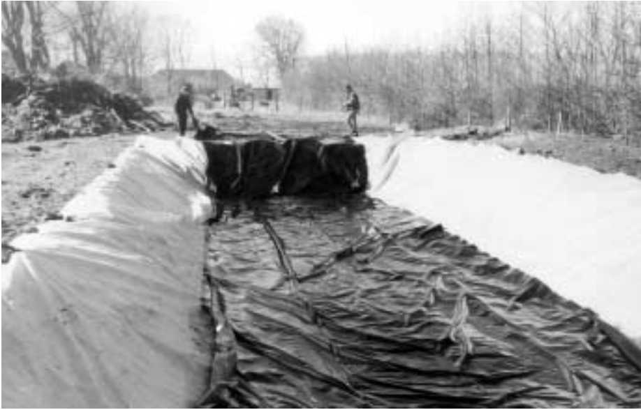
Figure 2 Excavation for establishment of willow wastewater cleaning facility showing placement of geotextile and high-density polyethylene membrane
