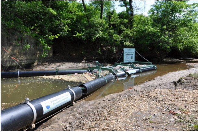
Figure 2: Bandalong trash trap installed on Watts branch, Washington DC.
