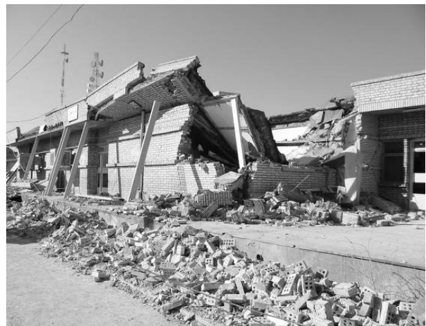
Fig. 2 Hospital building demolish because of depressed corner (photo by researcher).
