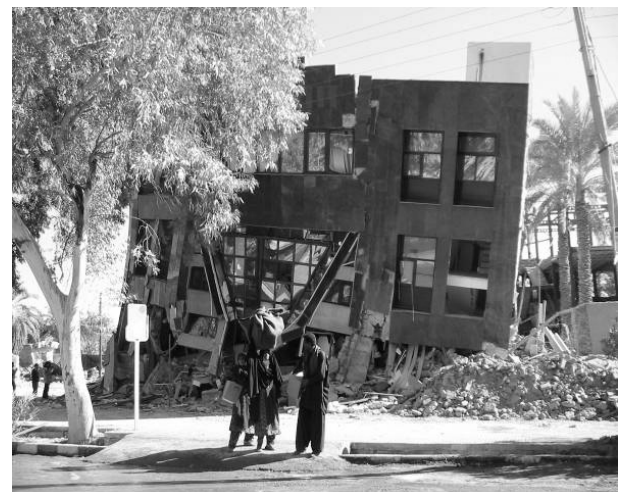
Fig. 6 Demolition of Kimia building because of the first soft story and short half-story column, Bam earthquake (photo by the researcher).
