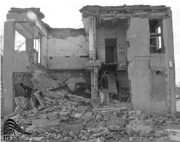
Fig. 5 Total destruction because of opening in diaphragm, Zarand Earthquake [8].
