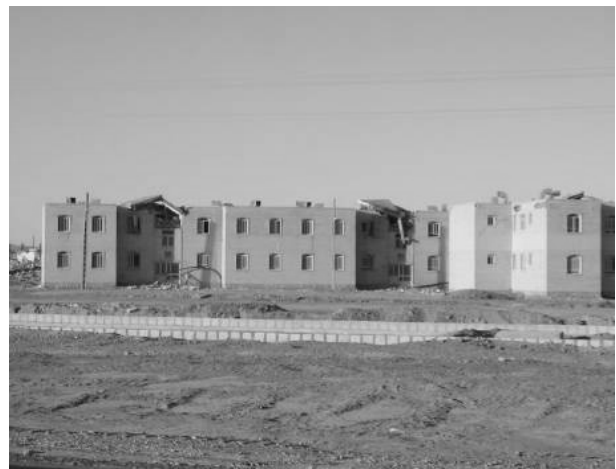
Fig. 8 Damage of building's mound, Bam earthquake (photo by the researcher).
