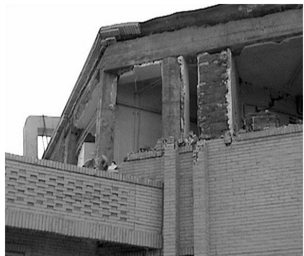
Fig. 4 Unparallel system, Bam earthquake [7].
