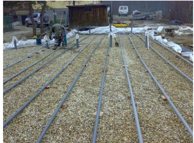
Figure 7. VF constructed wetland at Bojna, Slovakia. Photo courtesy F. Reffesberg.
