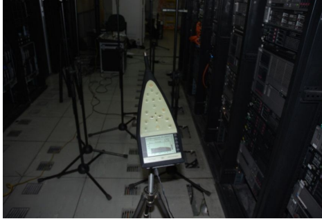
Figure 3. Measuring the acoustic noise characteristics in IRIB data center by using investigator 2260.
