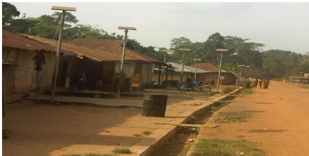
Figure 2. Installed solar street lights in Oke-Agunla, Ondo State, Nigeria.
