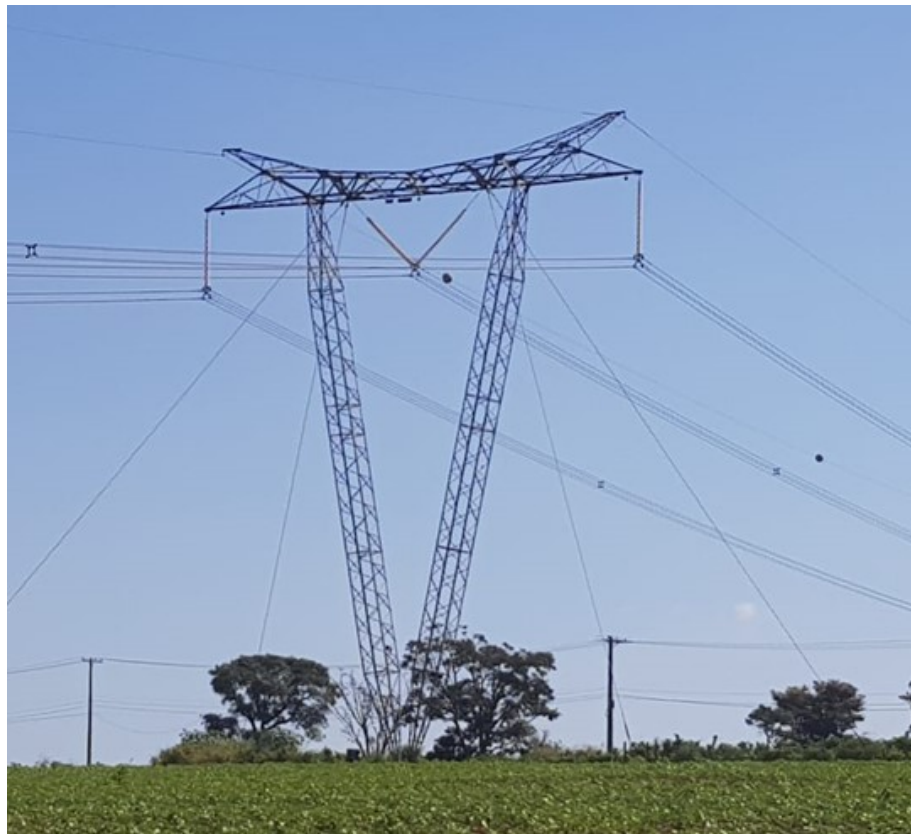
Figure 1. Typical guyed-V steel lattice tower commonly seen in the Brazilian power grid.
