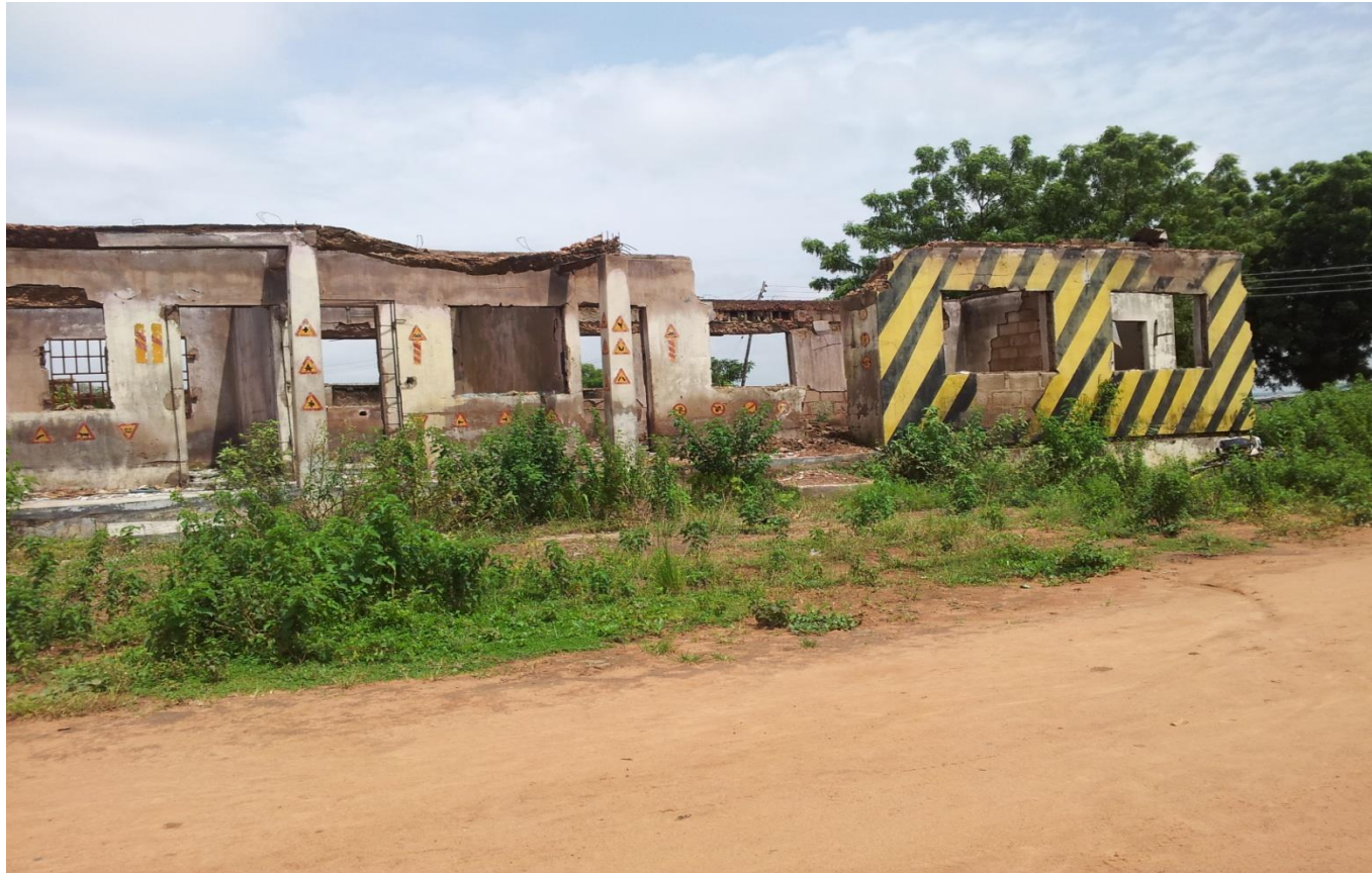
Vehicle inspection office razed by protesters
