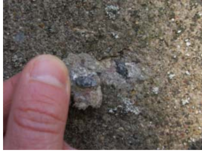
Fig. 5 A blistering piece of render on Building 47, with a large grey particle underneath
