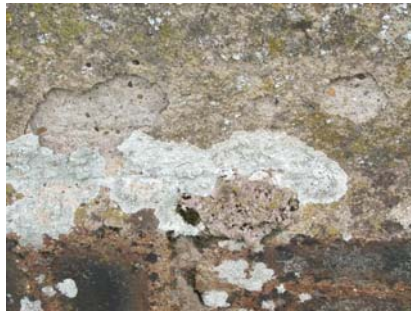
Fig. 2 The blistering render on Building 47 (Spare Parts Store)
