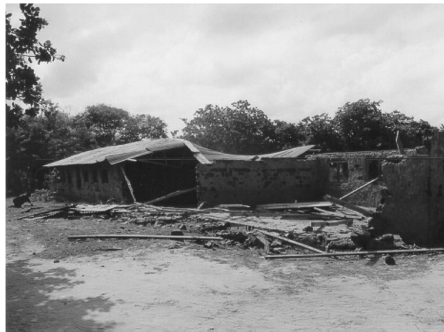
Figure 2 A Building That Collapsed During the Performance of a Study in Rural Tanzania
