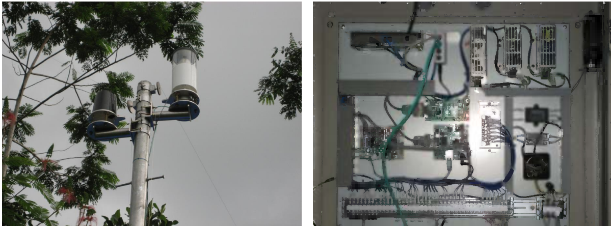
Fig. 2 The fixed pole with rain gauge and network camera, and the outdoor box with Fieldserver and other associated circuits
