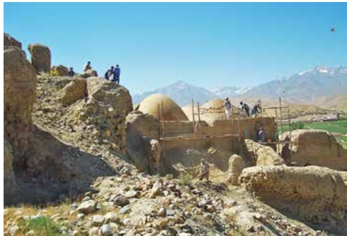
Construction work at the fortress of Shahr-i Ghulghulah at the Bamiyan World Heritage Site, Afghanistan. Photo courtesy of MACCA.
