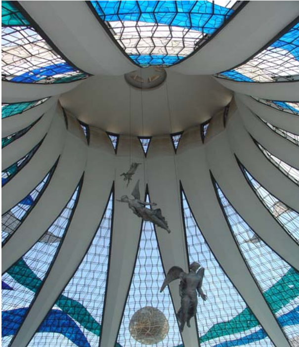
Fig. 7 Brasília Cathedral, present state: view towards detail of the compression ring, roof slab and glazed curtain walls among the piers.
