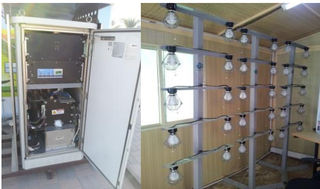
Figure 1: The ElectraGen™ PEMFC system and the 3 kW Load.
