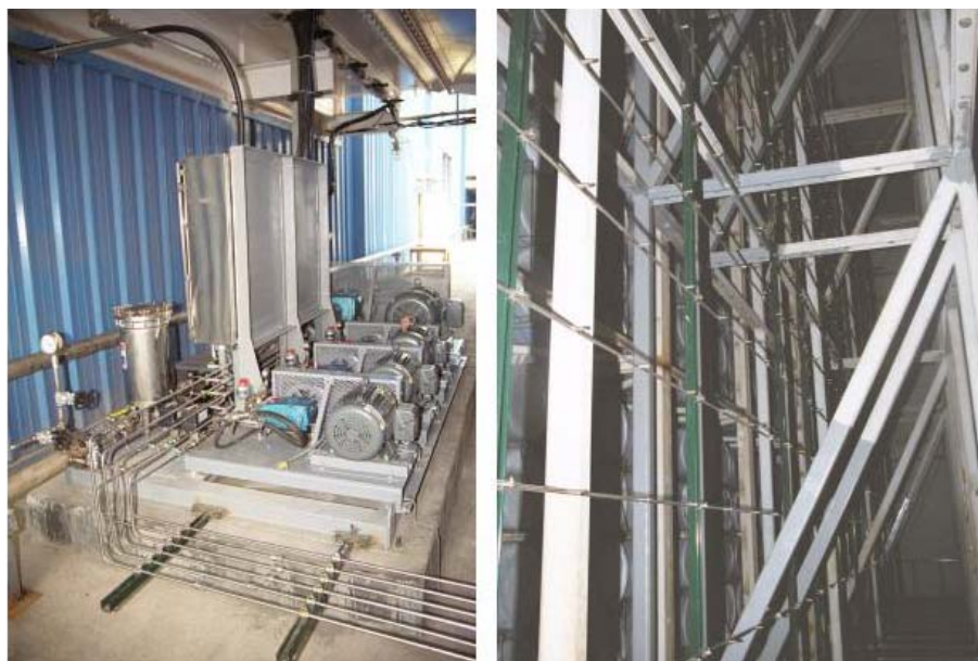
Figure 2 – A fogging nozzle array inside a GE 9FA filter house (right) and a high-pressure fogging pump skid (left). Photos: American Moistening Co., Pineville, NC
