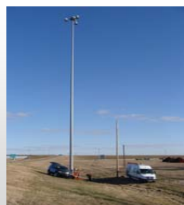
High Mast Lighting Tower (HMLT)
