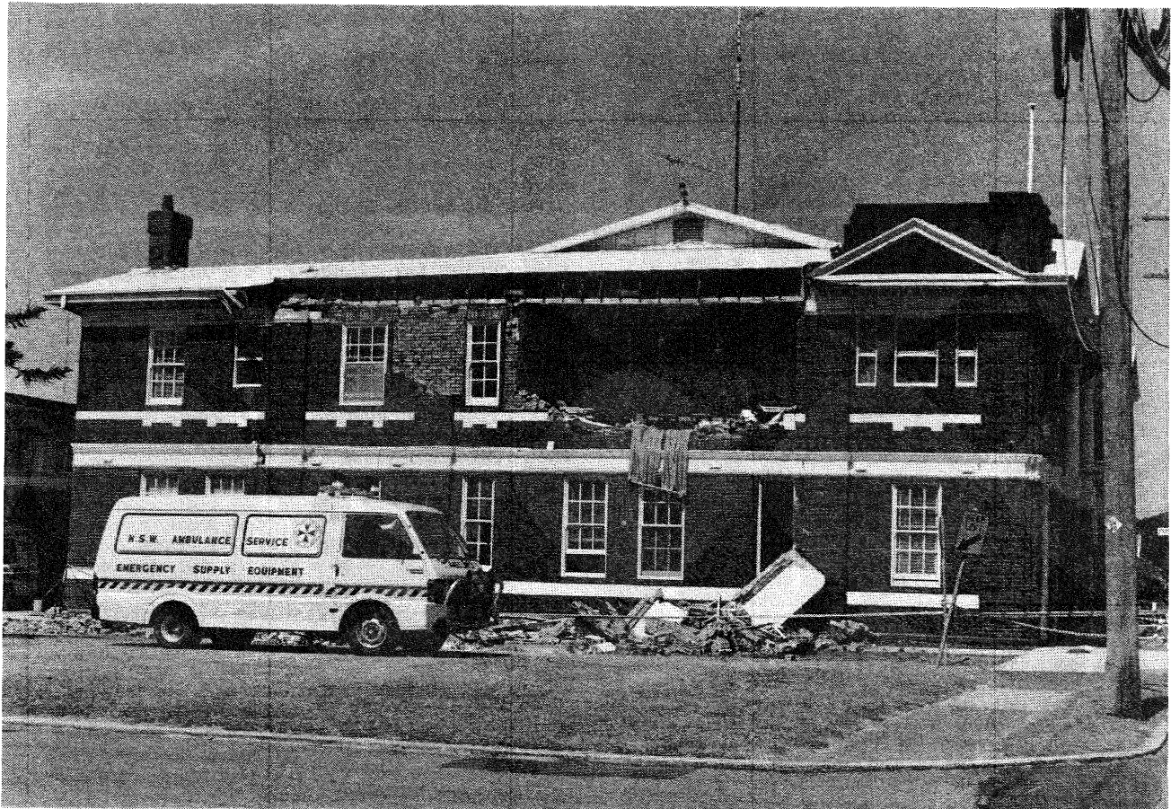
FIGURE 12 DAMAGE TO REGIONAL AMBULANCE HEADQUARTERS, HAMILTON.
