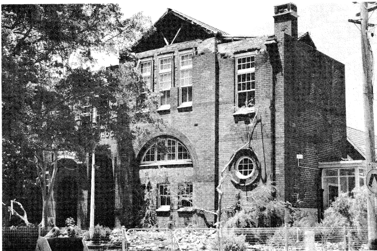
FIGURE 8 GABLE END FAILURE - THE JUNCTION SCHOOL
