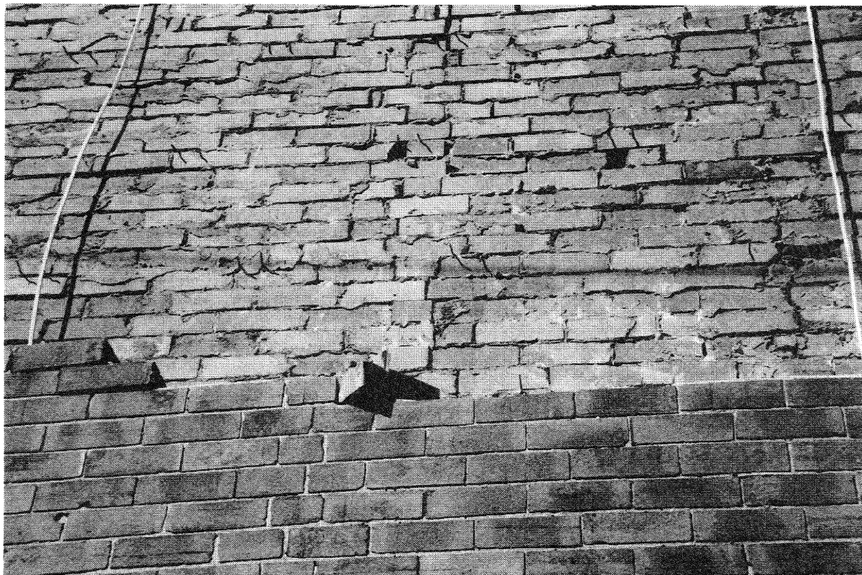
FIGURE 10 CORROSION OF BRICK CAVITY TIES
