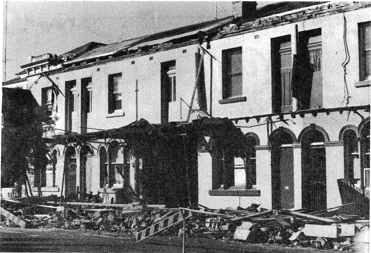
FIGURE 6 PARAPET AND AWNING FAILURE - RESIDENTIAL BLOCK
