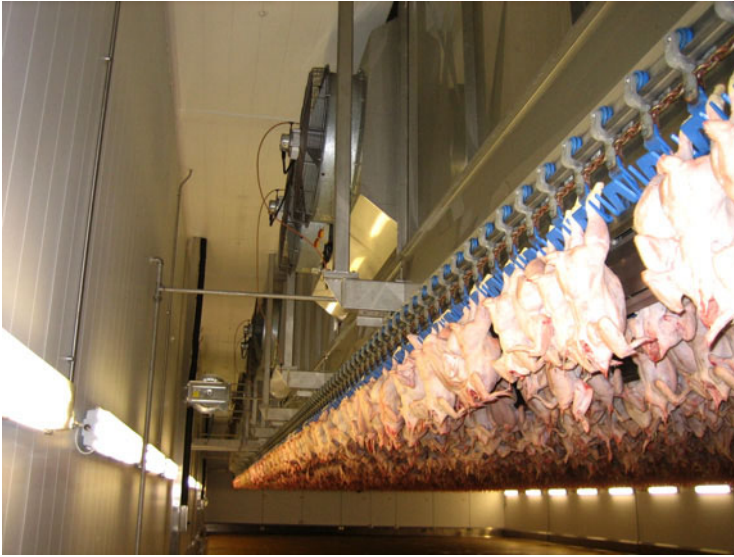
Figure 5.3 Continuous air-chilling system for whole poultry carcasses.
