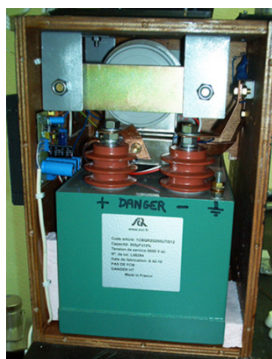
Figure C-3. Power box. The Energy storage capacitor C of 206.5 \mu F value is the large green lower volume. It is insulated to 5000 Volts. The power thyristor (Dynex PT85) is installed over it. Insulated to 3000 Volts, it is capable of 20 k Amperes discharge current. On the left side is the electronic / optical relay for triggering the thyristor, from a safe distance, by wire manual command. Components are connected by 50 mm 2 Copper bars. A Rogowski coil sensor plus its passive integrator allow the discharge current measurement. On the front panel (right side) is the four digits calibrated voltmeter, measuring the charge voltage U_0 of capacitor C
