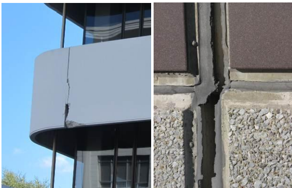
Figure 9: Corner crushing of spandrel panels (left), torn polysulphide seal (right).
