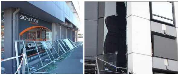
Figure 2: Examples of heavy damage to facade systems caused by the February 22 earthquake.
