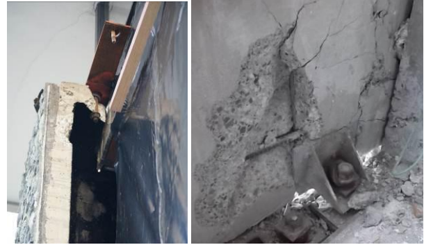
Figure 10: Connection of coffered precast panels that failed in June 13 aftershocks (left), precast panel and connection damage due to beam elongation (right).
