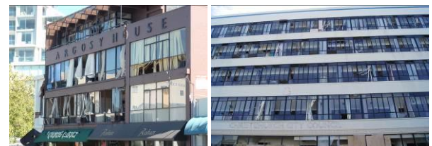
Figure 11: Damage to light-medium weight cladding.
