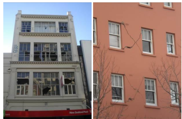
Figure 14: Examples of damage to infill systems.
