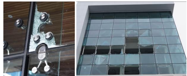
Figure 13: Examples of damage to spider glazing systems.
