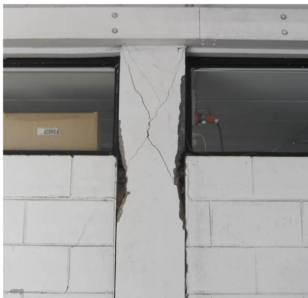
Figure 15: Short column effect due to infill.
