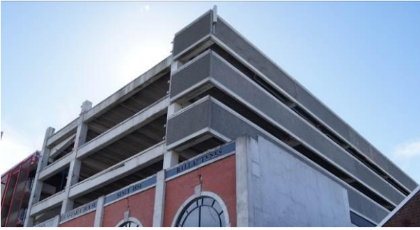
Figure 8: Structure with disconnected spandrel panels.
