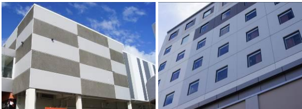
Figure 3: Examples of heavy cladding present on Christchurch buildings.
