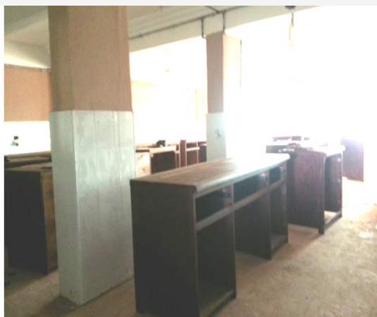
Figure 9: Showing columns misallocated in the middle of a classroom hall interior of an elementary school built in Sharkeya province of Egypt, regardless the violation of this solution to the simplest architectural classroom design standards.
