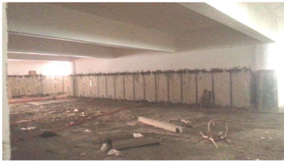
Figure 11: Showing the interior of a multipurpose hall under construction in the Sharkeya province of Egypt. where all ceiling beams depths exaggerated leaving the hall with a clear height close to the lentic heights of its entrance doors.
