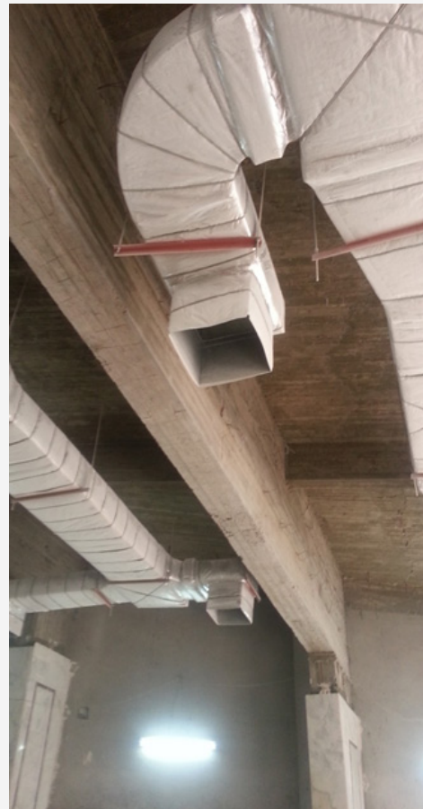
Figure 13: Showing HVAC and Electromechanical works interference with the ceiling girders in the same multipurpose hall of Sherkeya province, Egypt.
