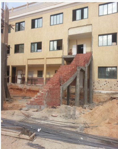
Figure 12: Showing a large external stair case added to the façade of the same school in Sharkeya province, Egypt.
