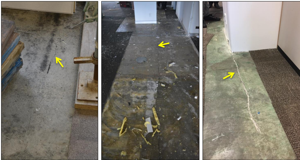
Figure 6: Examples of cracks in floor topping.
