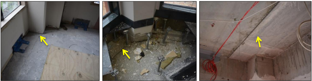
Figure 8: Damage in corners of floor diaphragm – Single cracks.
