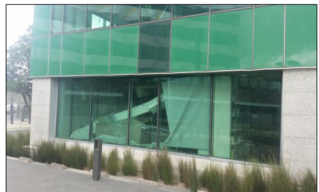
(b) Collapsed floor unit in corner of ground floor
