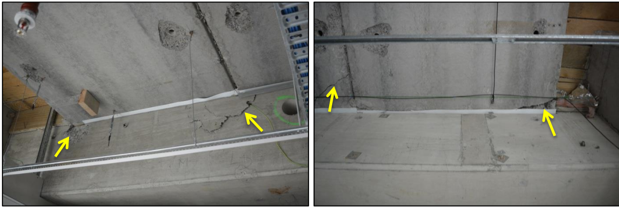
(a) Spalled support beam
