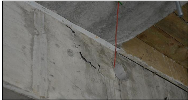
(b) Minor spalling (with low-friction strip)
