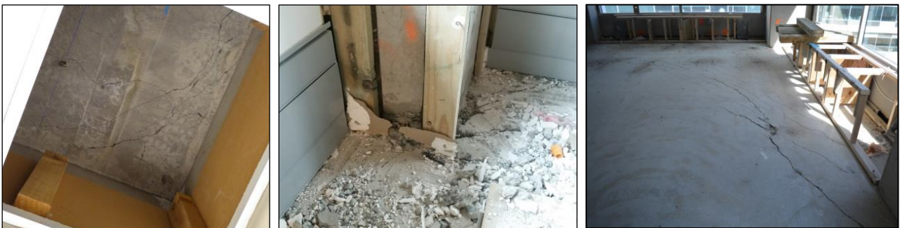
Figure 9: Damage in corners of floor diaphragm – Significant cracking.
