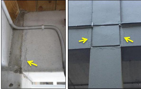
(a) Minor cracking
