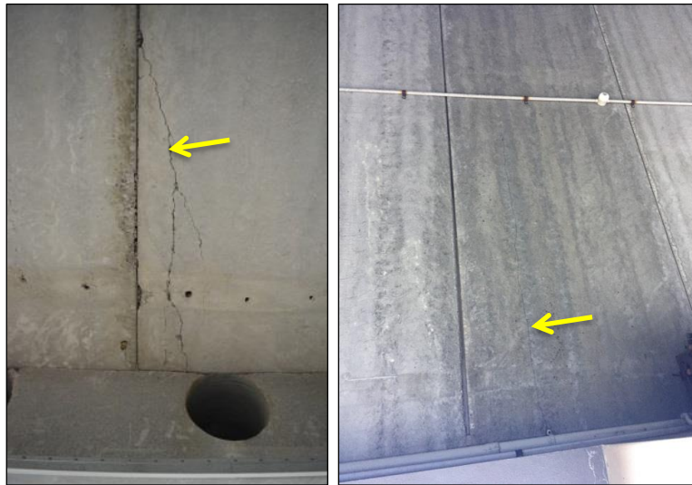
(a) Cracks only at ends
