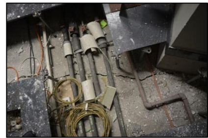
(b) Wide floor cracks
