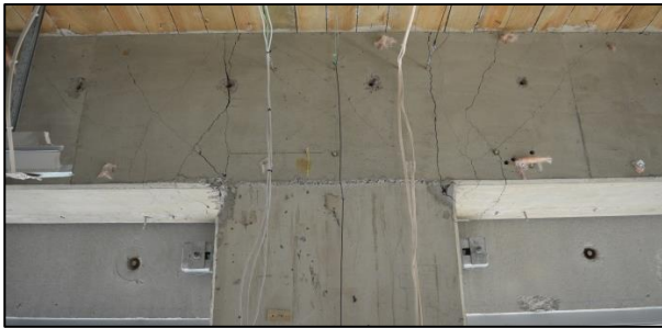
(b) Moderate cracking
