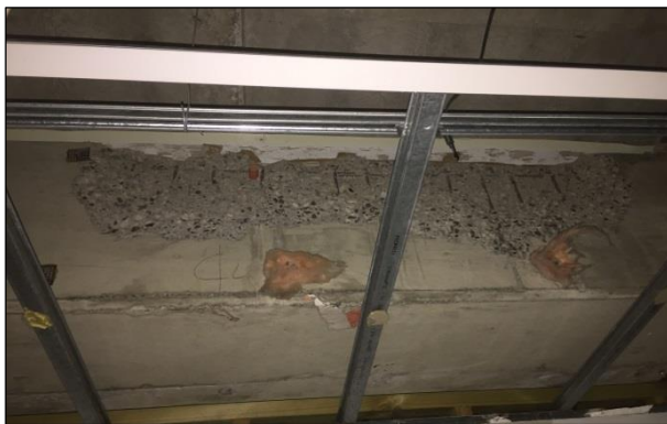
(c) Spalled ledge exposing reinforcing
