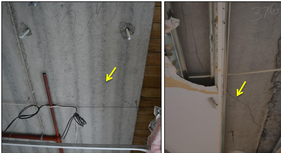
Figure 17: Diagonal cracks in hollowcore floor units.
