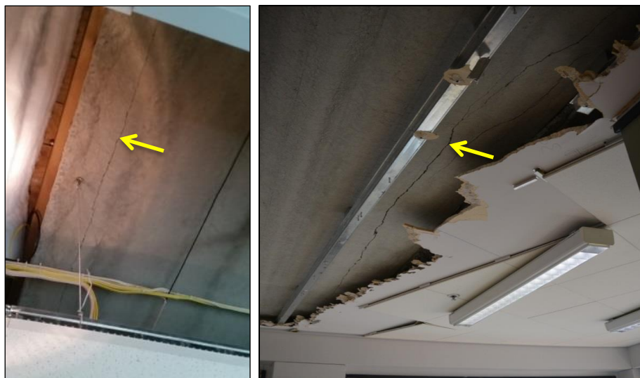
(b) Wide cracks along entire length
