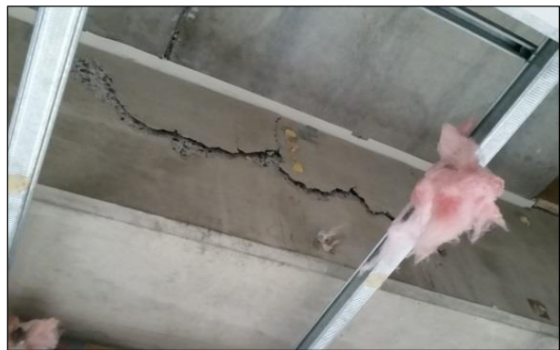
(d) Deep crack at support ledge with concrete still in place
