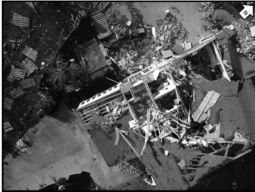
Figure 4. UAV-based still image of Structure 1 taken by the nadir-mounted digital camera, with GSD approximately 0.007 m.
