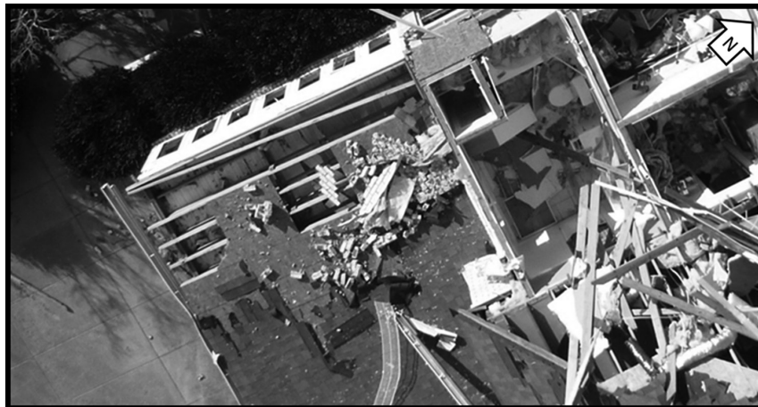
Figure 5. Close-up image of the southwest corner of the Structure 1, which is from the same image file shown in Figure 5, but shown at a higher zoom. While some roof decking has been removed from the edge, ceiling joists are largely intact for the single story exterior corner room in the top left of the image, while the entire roof and ceiling structure has been removed from the adjacent second floor rooms in the top right of the image.
