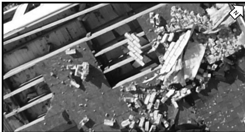
Figure 6. Further close-up of the southwest corner of Structure 1. This image is from the same imagery files shown in Figures 4 and 5 displayed here at an even higher zoom, which demonstrates the full resolution capabilities of the UAV-mounted camera. Construction materials, and damage to the roof covering, roof sheathing, and ceiling beneath the roof joists are clearly visible.
