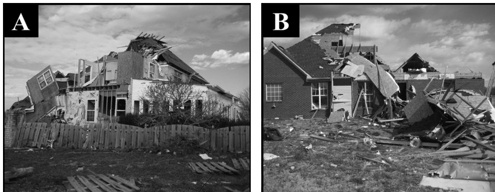
Figure 3. Ground-based imagery of tornado-damaged structures of interest: (A) southwest facing elevation of Structure 1, a heavily damaged two-story home. The fence and unstable nature of the significantly damaged structure prevented close-range ground-based investigation. (B) West facing elevation of Structure 2, a severely damaged one-story structure. The extent of damage beneath the roof line is difficult to quantify based on this ground-based imagery.
