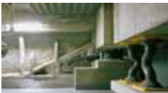
Interior view of isolation layer • Natural rubber laminated rubber isolators 800φ: 40 No. • 180φ lead dampers: 212 No.
