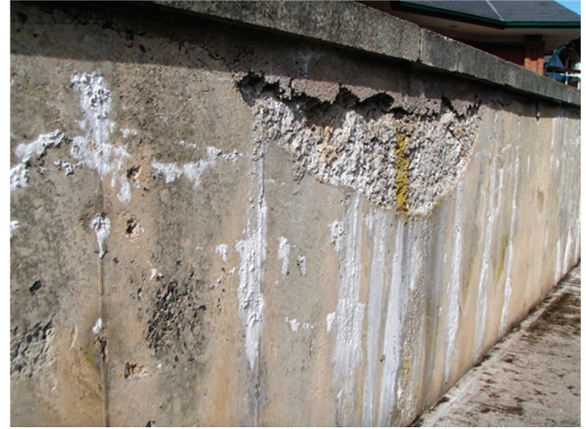
Spalling of concrete cover layer (courtesy of the Environment Agency).
