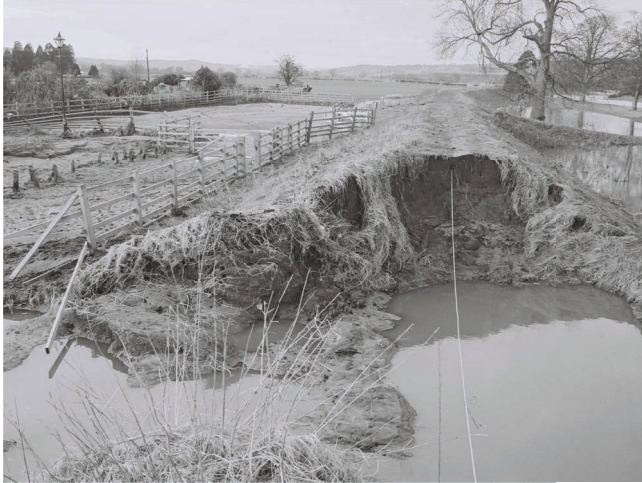
Flood defence embankment breaches following high water levels at Corbridge in Northumberland (courtesy of Mike Walkden, 10 January 2005).
