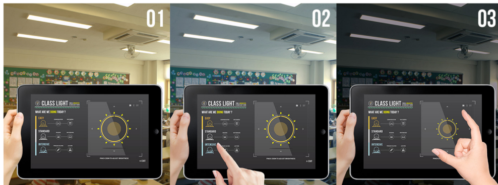
Fig. 6. Operational flow of the dynamic lighting system: 1) students are focusing on solving mathematical problems; 2) select the “intensive” lighting preset to support students’ academic performance; and 3) lower the illuminance level by pinching in the intensity icon for high intensity of daylight.
