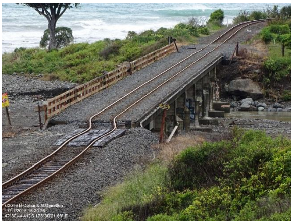
(e) Rail bridge 97 MNL approach offset and rail alignment failure. Photo credit: Dizhur & Giaretton
