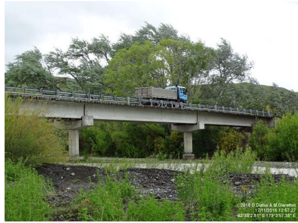
(b) Lower Mason bridge with damaged supports. Photo credit: Dizhur & Giaretton
