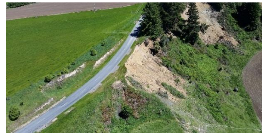
(b) Landslide undercutting road, slumping potential. Photo credit: Aurecon, 2016
