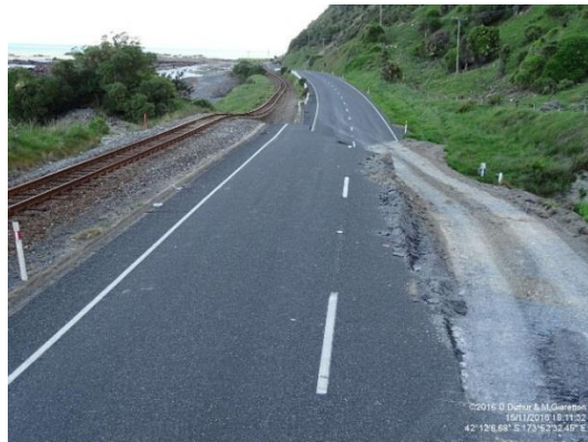
(b) Pavement rupture due to fault rupture and subsequent access ramp. Photo credit: Dizhur & Giaretton
