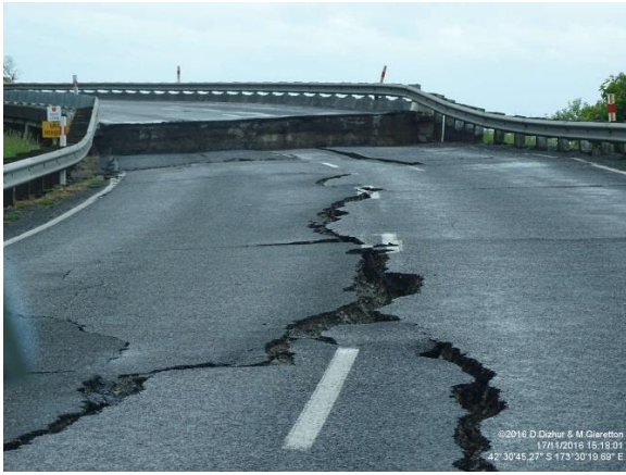
(a) Oaro bridge approach failure and pavement cracking. Photo credit: Dizhur & Giaretton
