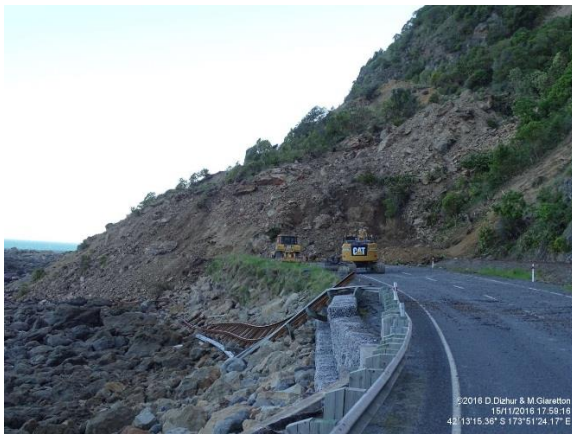
(c) Large offset of rail track due to landslide Photo credit: Dizhur & Giaretton
