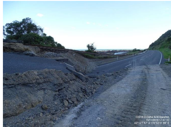
(b) Rail line suspended by fault rupture (angle 2). Photo credit: Dizhur & Giaretton
