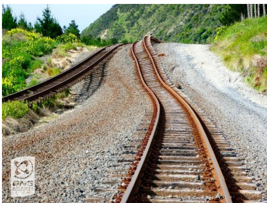
(e) Rail tracks severely distorted and misaligned due to fault rupture. Photo credit: William Ries, GNS Science
