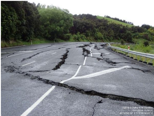
(a) Pavement cracking on SH1 due to slope instability. Photo credit: Dizhur & Giaretton
