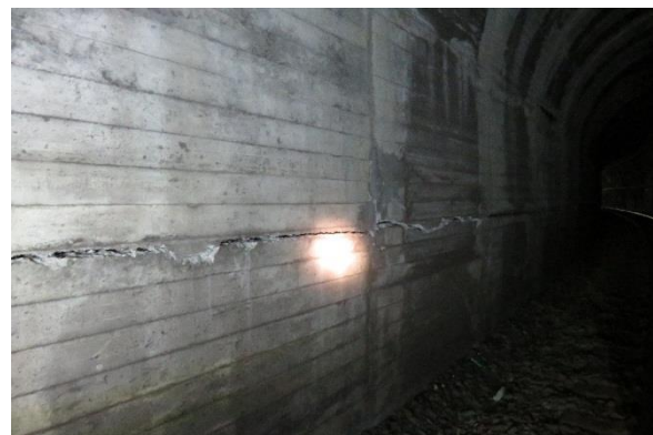
(f) Cracking of tunnel wall. Photo credit: KiwiRail.
