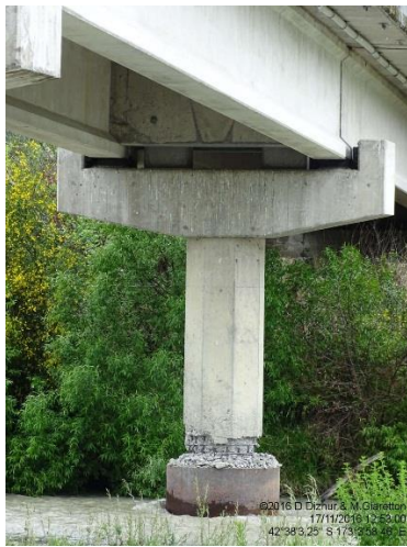
(c) Lower Mason bridge support damage. Photo credit: Dizhur & Giaretton
