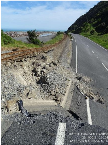
(a) Rail line suspended by fault rupture (angle 1). Photo credit: Dizhur & Giaretton
