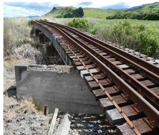
(f) Rail bridge 129 MNL span dislocated from abutment due to Kekerengu Fault rupture. Photo credit: Tim Little, VUW.
